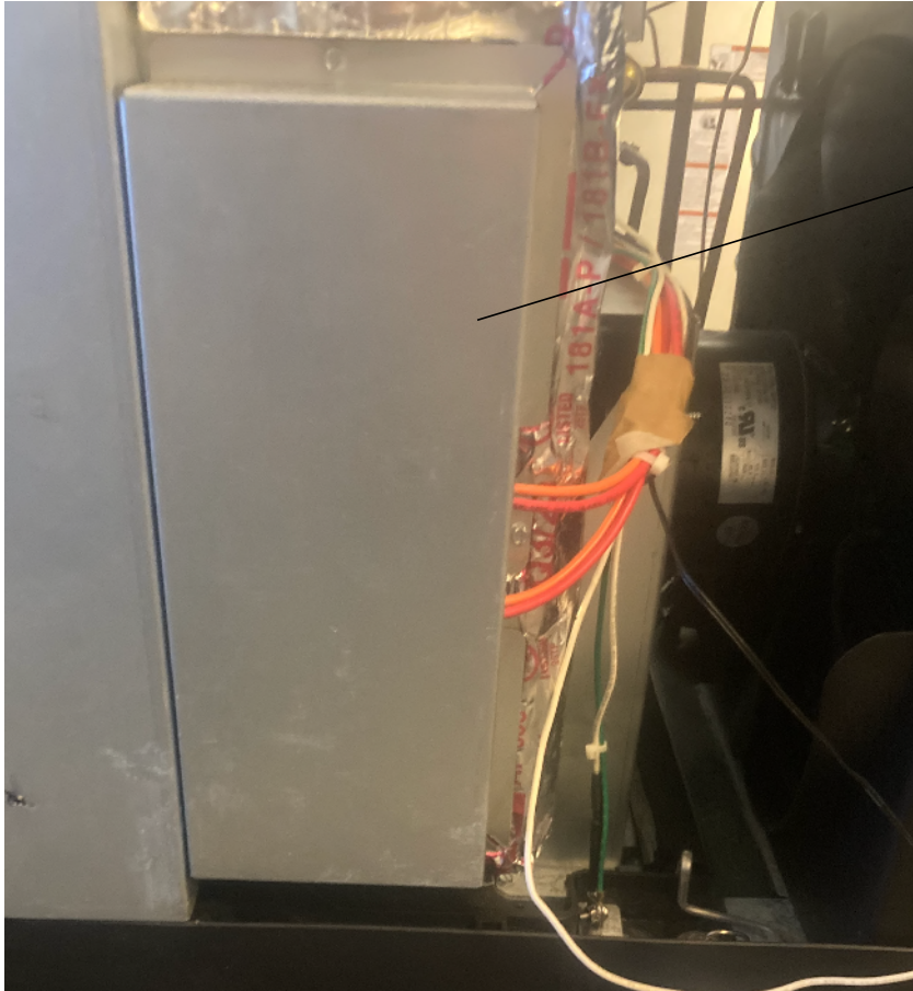
Heater Access Panel
